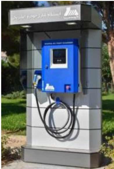
Fast Wall-box Charger
