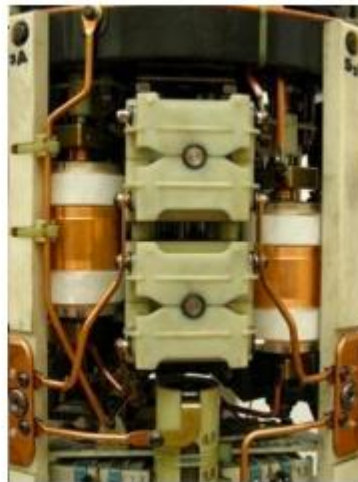
Tap-Changer after 300,000 operations
