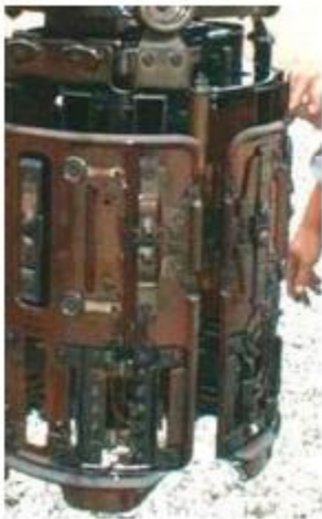
Tap-Changer after 80,000 operations
